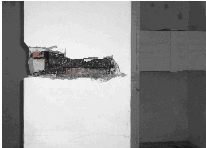
Fig. 5. “In-situ” inspection hole of the steel supporting structure of the column. Visible degree of column corrosion
