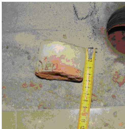
Fig. 1. Measurement of the thickness of the concrete slab – the overlayer of the Ackerman block ceiling
