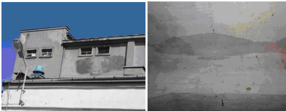
Fig. 8. The examples of the moisture-caused damages of the cold storage structural elements
