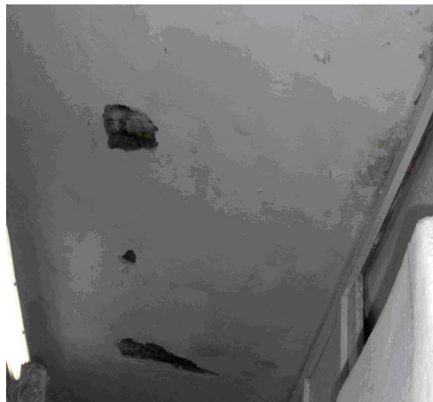
Fig. 4. “In-situ” inspection hole of Klein ceiling beams in the cold store in Warsaw
